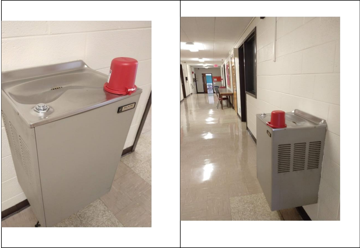
Second floor FST inactive water bubbler located across from Sensory kitchen that is used by student organizations and undergraduate courses. Classroom FST 132 is pictured at the end of the hall.
