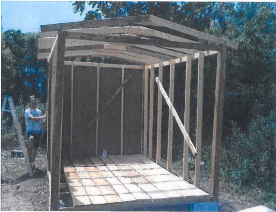
Summer 2012 - Midway through the construction of a shed as part of a Civic Agriculture Minor's capstone project. The shed is currently completed and will be painted in October 2012.
